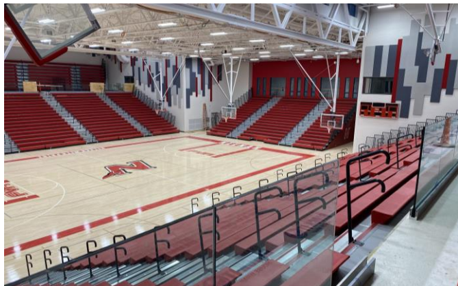
Lower bleachers are installed in the competition gym 03/30/2023
