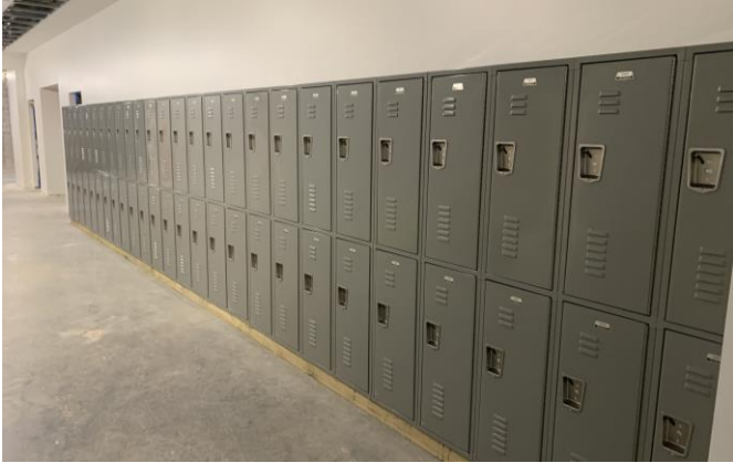
Academic lockers are installed 03/09/2023
